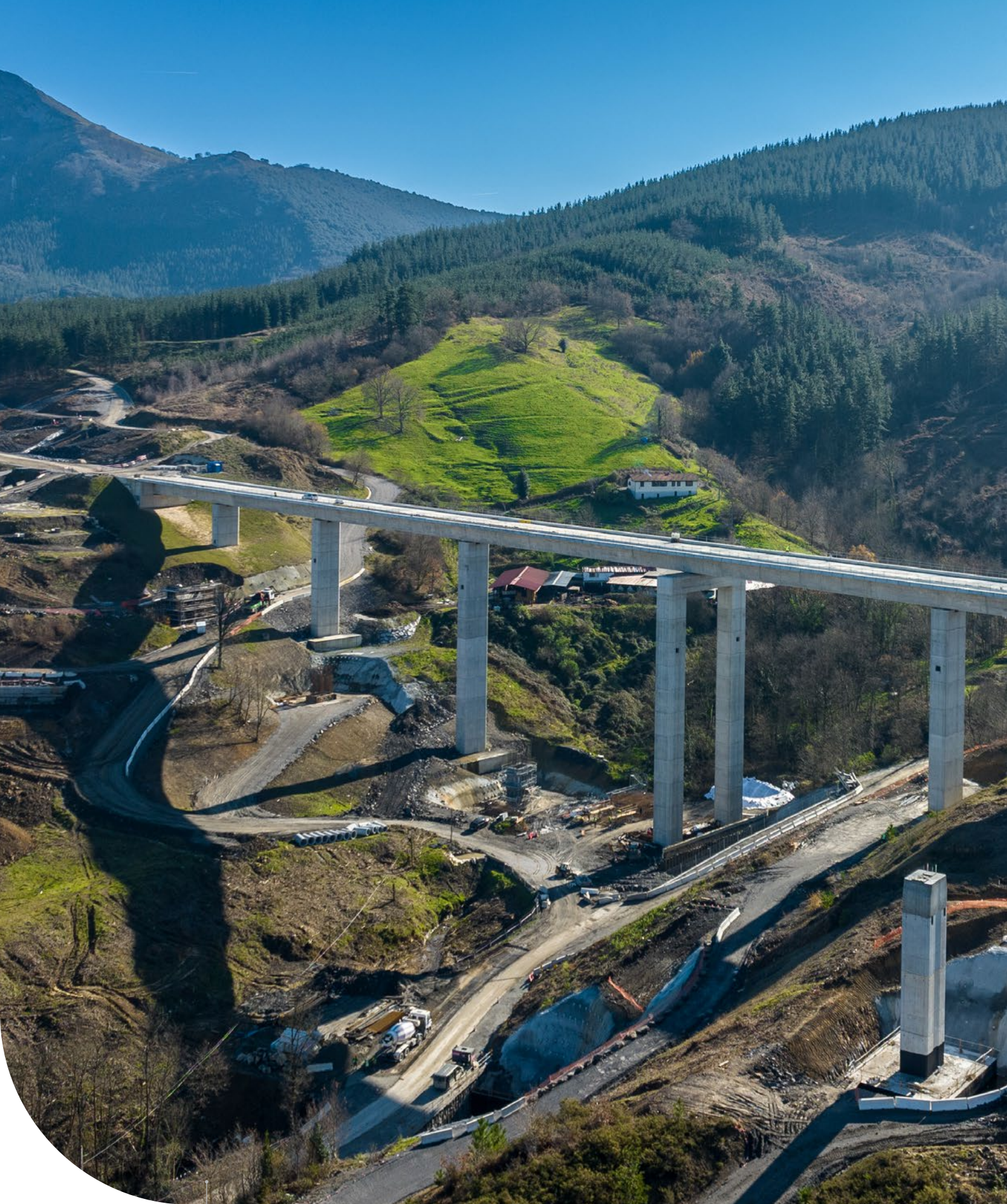
Image of the construction process of the UTE Elorrio project in Vizcaya.
